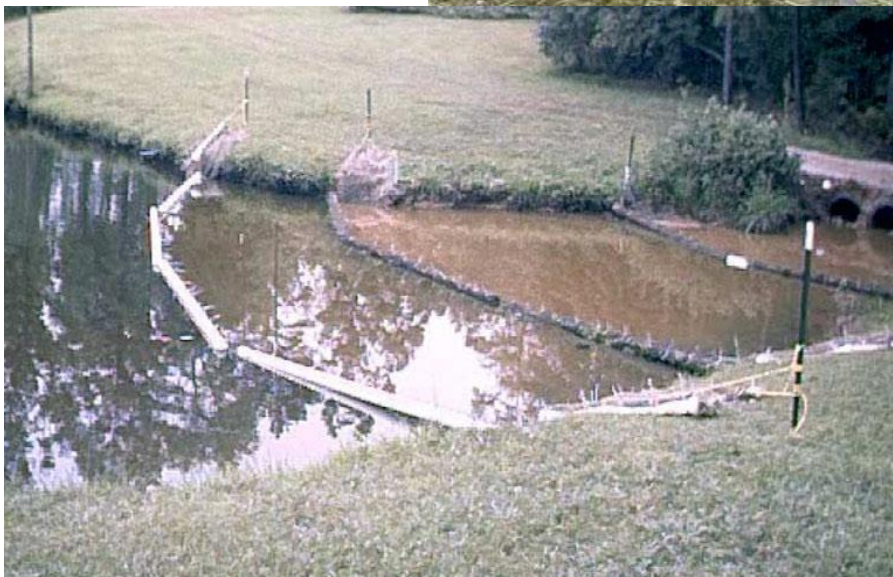
(Left) A series of particle curtains collect suspended flocculated material resulting in progressively clearer water.
